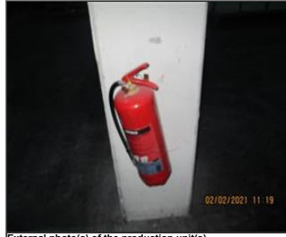
External photo(s) of the production unit(s) fire extinguisher.jpg
